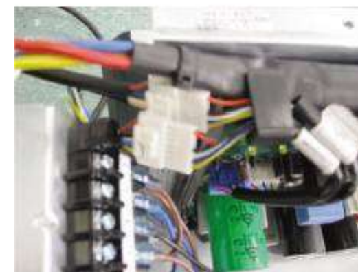
<fan motor middle connection>
